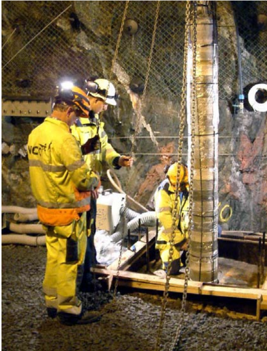
Installation of one of the packages illustrating the mixing of the different compacted buffer discs.
